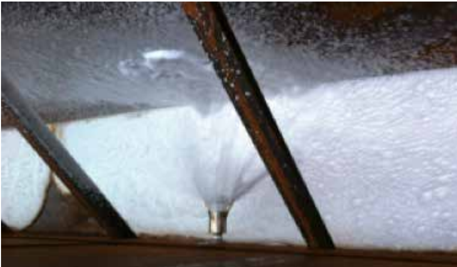
AFFF Foam based unit spraying in between primary and secondary seal for vapor sealing purpose.
